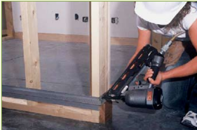
Figure 4-1: Using nails with a nail gun is the fastest way to fasten the UMB to wood.
